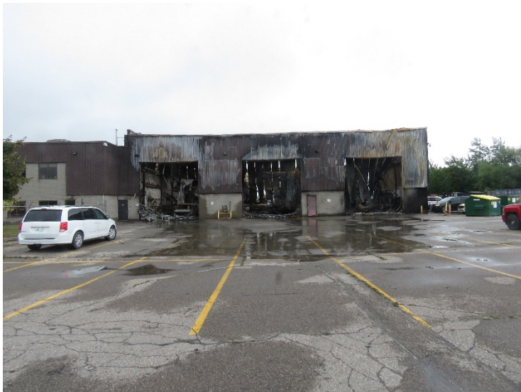
Front of the section of the building where the fire originated
